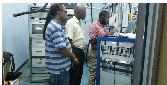
Top image: Mr. Edwards and Ing. Carr training at Cable AML. Bottom image: ABS TV team installing transmitter on site.
