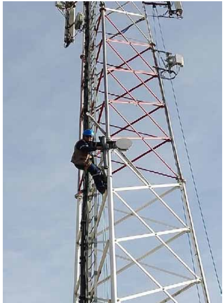
28 GHz Repeater installation
