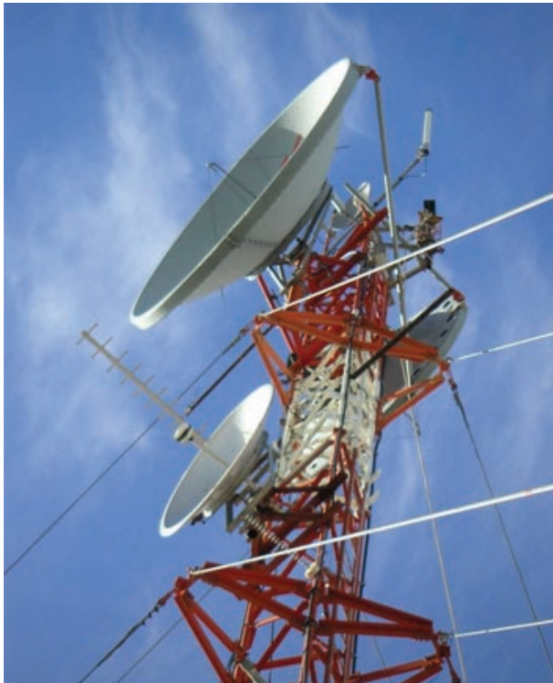
Wireless return Path Antenna for DOCSIS Cable Modem Service is installed on existing tower next to PTP antennas.
