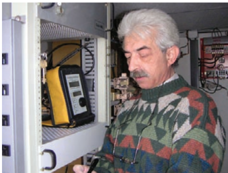
Horacio Indaco of Cablevision del Comahue installing the headend equipment for the Wireless DOCSIS return system provided by Cable AML.
