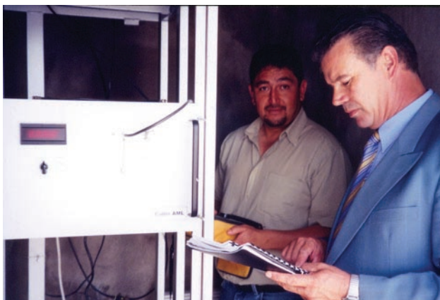
Randel Rivas and Armando Carrillo inspect installation of Repeater in Zacatecas, Mexico
