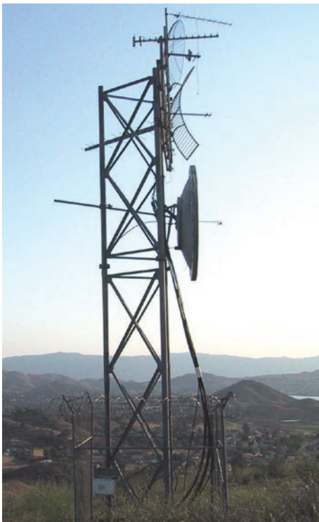
Mediacom off-air receive site.
