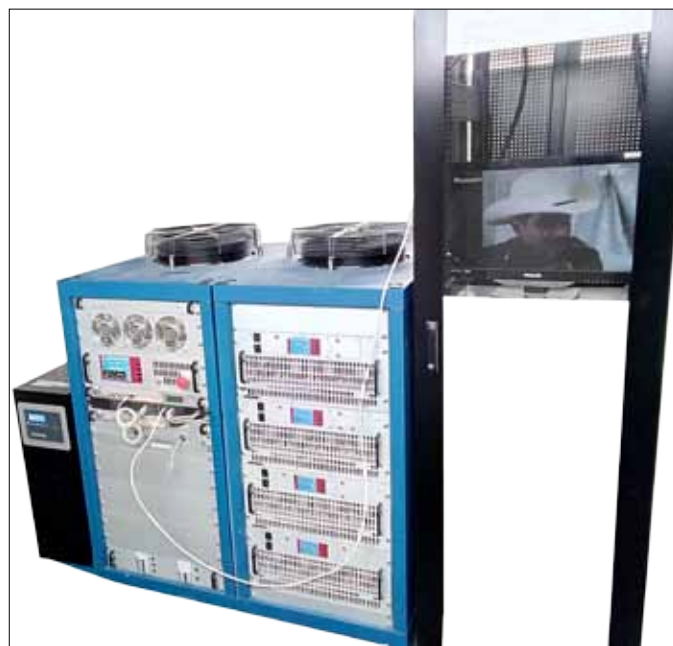
1.7 kW RMS Transmitter system and STL indoor receiver unit installed in Cerro la Virgen, Zactecas (Mexico)
