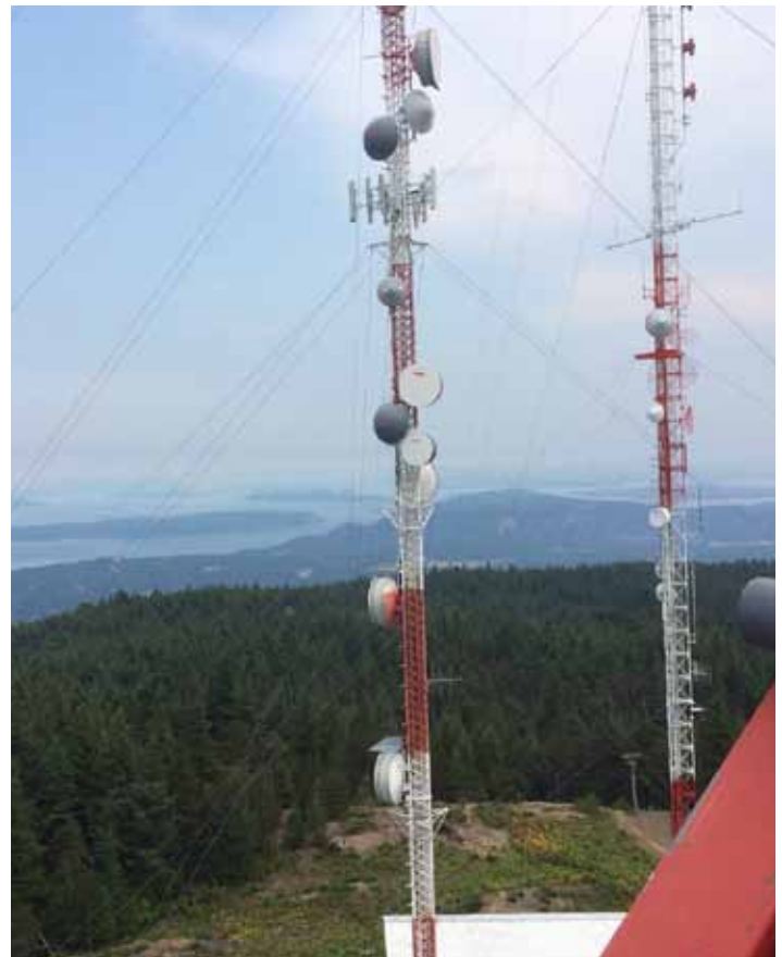
Microwave tower at Orcas Island, Washington, USA
